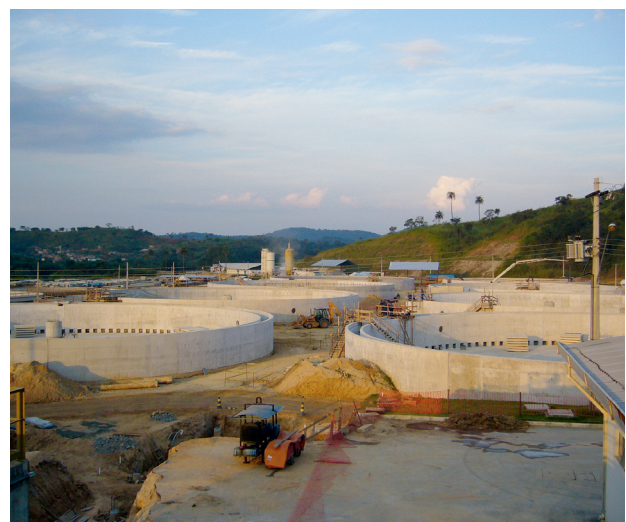
Construction of trickling filters at a sewage treatment plant in South America
